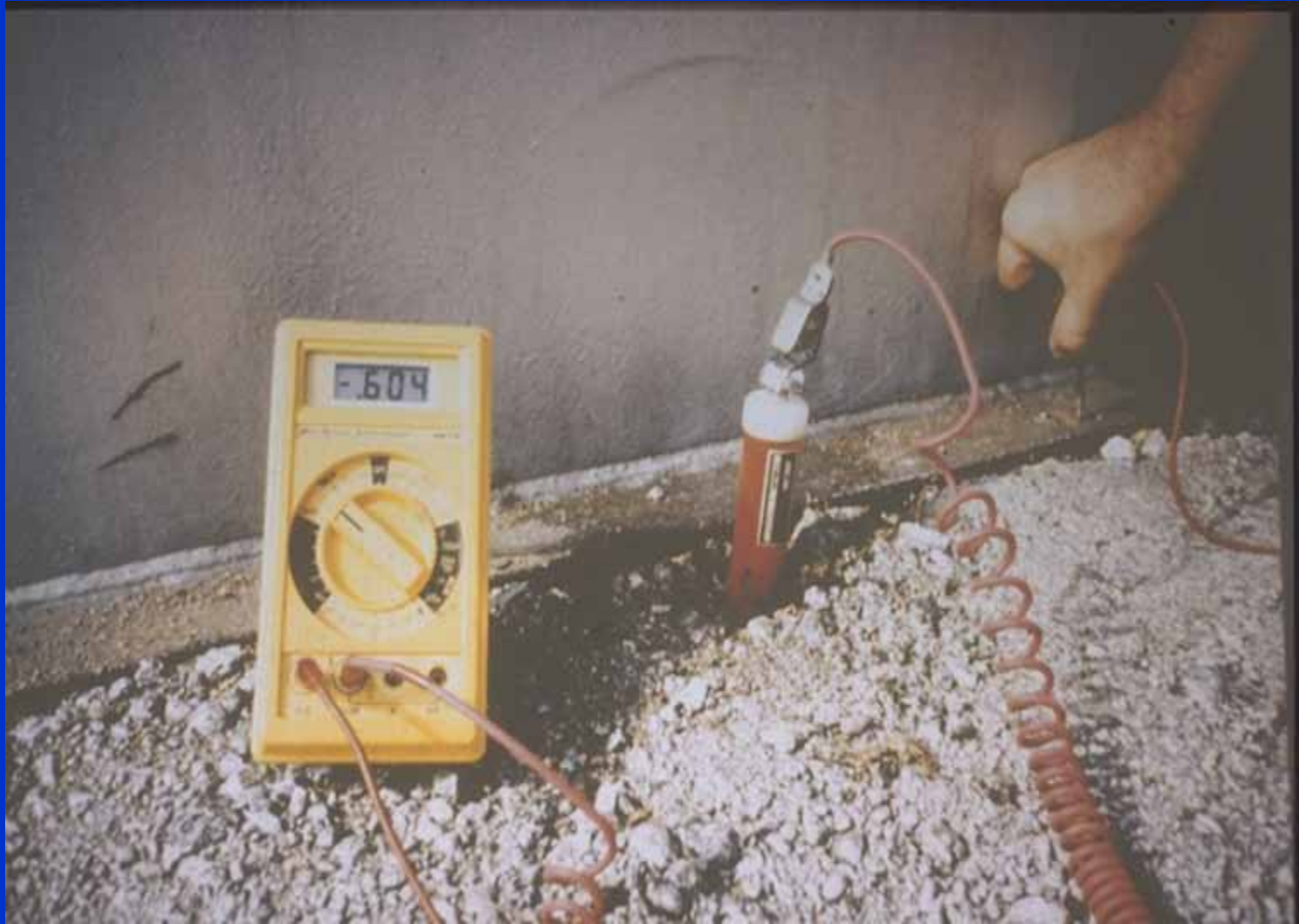
Tank to Soil Potential Measurements
