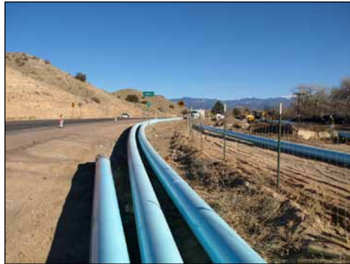
Fused pipe strands
